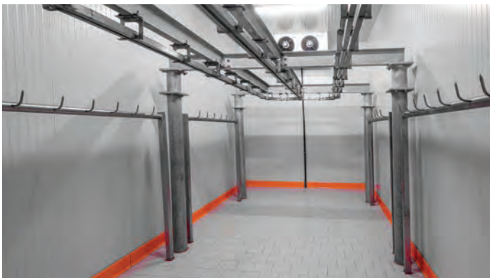
Cold Room and Storage
